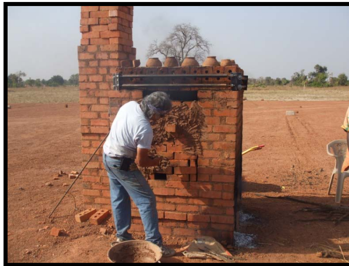
Sealing the Kiln Door with Brick and Mortar, Except for Upper Row of Bricks
