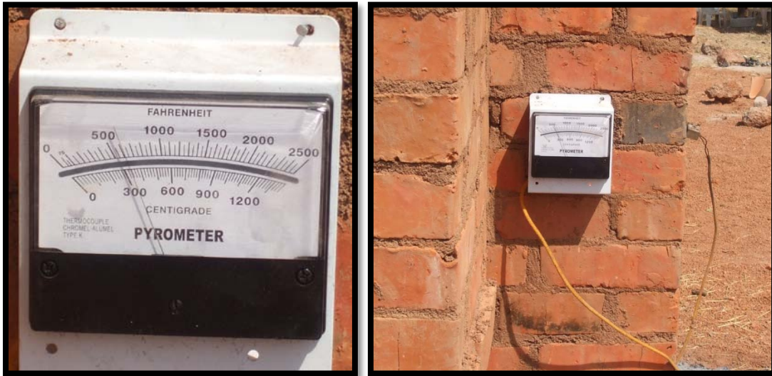
Left: Pyrometer Temperature Read-out, Right: Pyrometer Read-out with Wire to Probe
