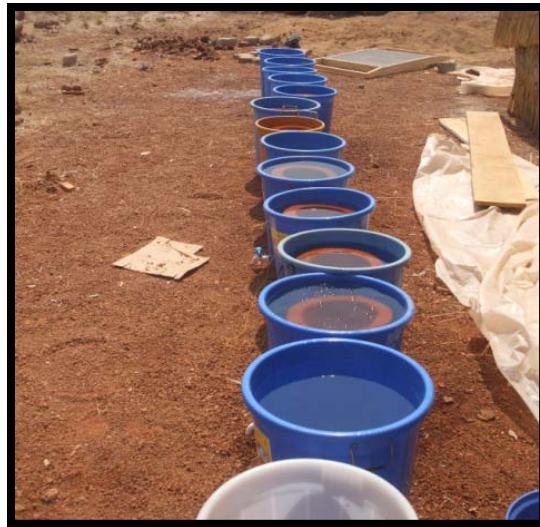
Filters Soaking with Municipal Water in Large Plastic Buckets
